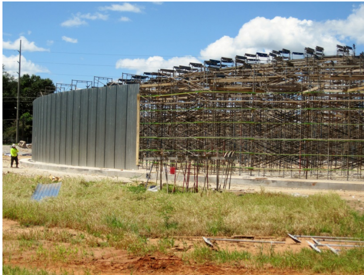
Photo: Bienville tank
