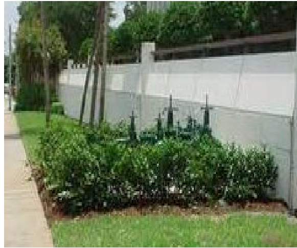
Bushes Screening Backflow Prevention Assembly
