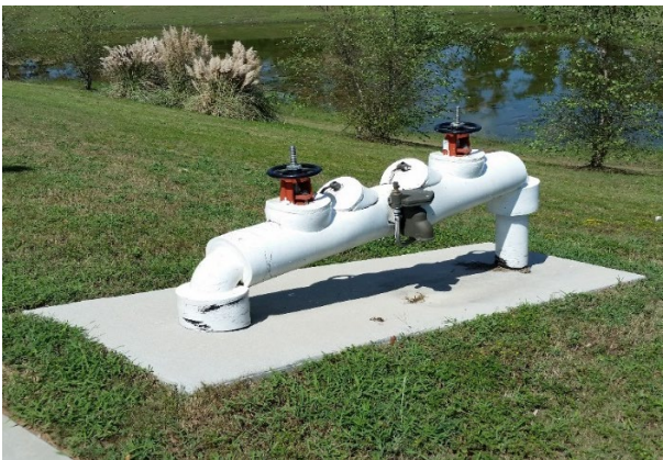
Double Check Valve with Pipe and Valve Insulation
