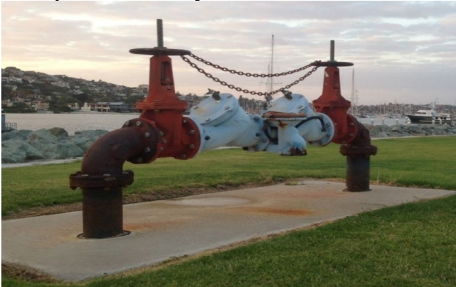
Double Check Valve Assembly with Secured Valves Operators
