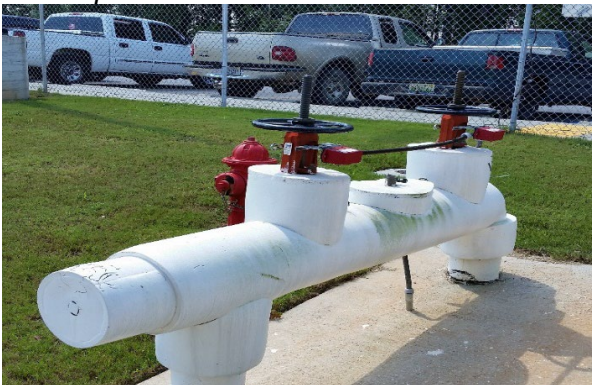
Double Check Valve with Valve Operation Alarm Switches and Insulation
