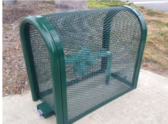
Residential Backflow Prevention Assembly with Locked Enclosure
