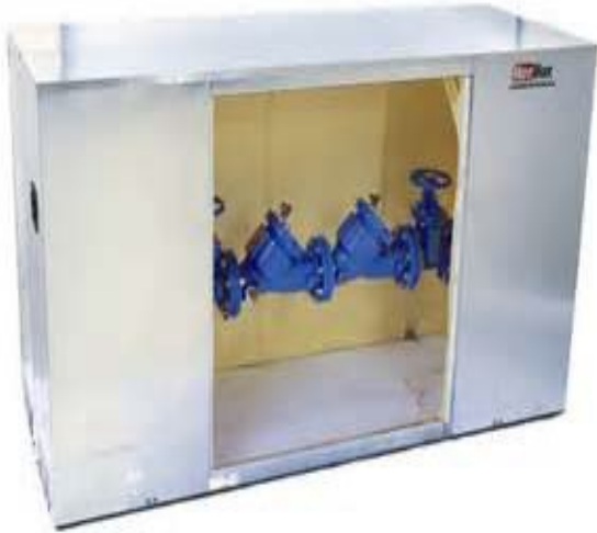
Freeze-protected Aluminum Enclosure Over Backflow Prevention Assembly
