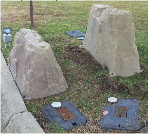
Faux Rocks Covering Backflow Prevention Assemblies
