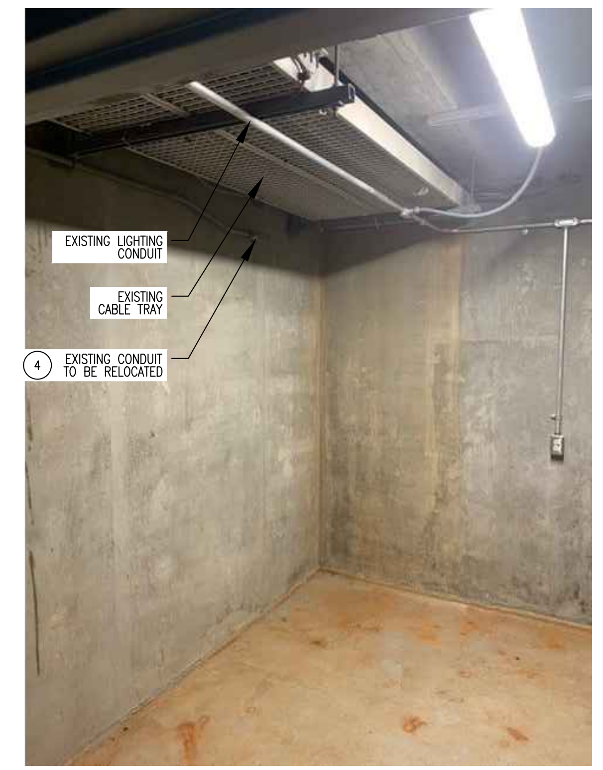
VFD ROOM PHOTO NO. 3 (WEST)
