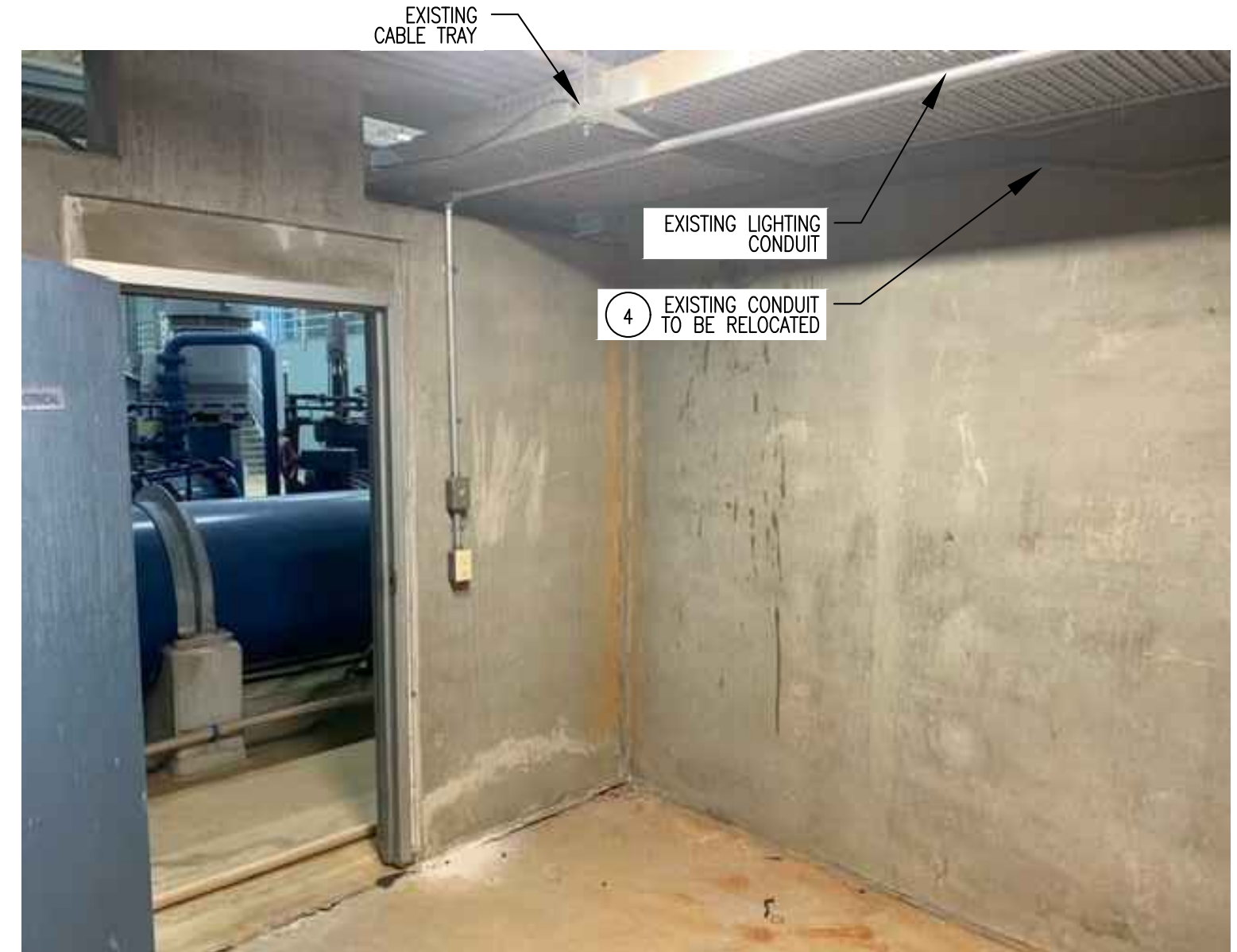
VFD ROOM PHOTO NO. 1 (EAST)
