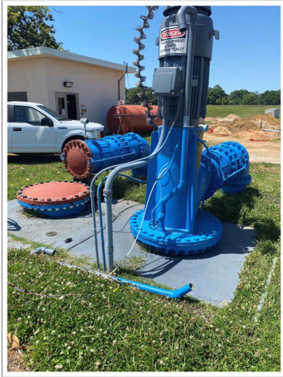
PHOTOGRAPH 3: EXISTING VERTICAL TURBINE PUMP AND DISCHARGE
