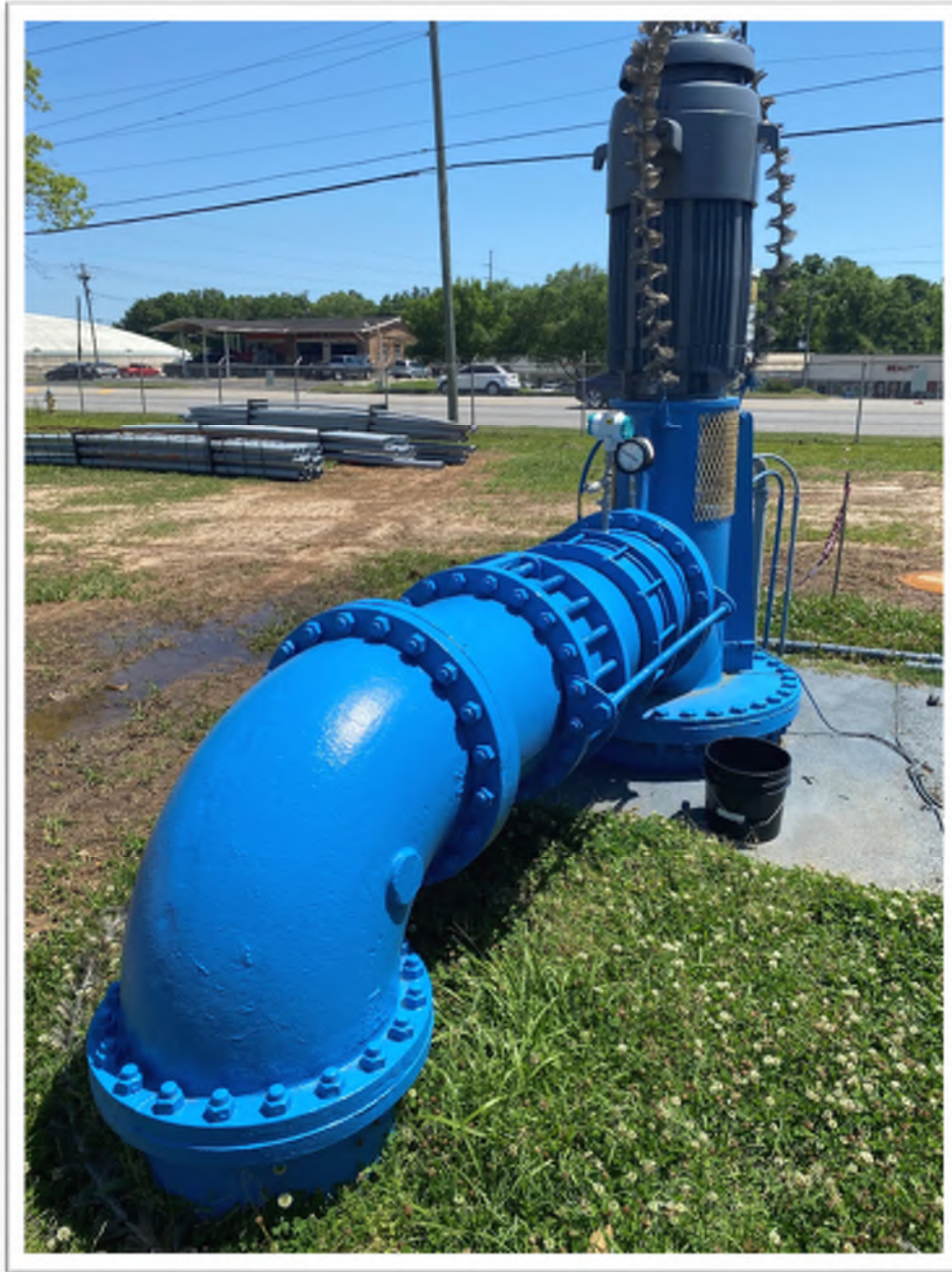
PHOTOGRAPH 2: EXISTING VERTICAL TURBINE PUMP AND DISCHARGE
