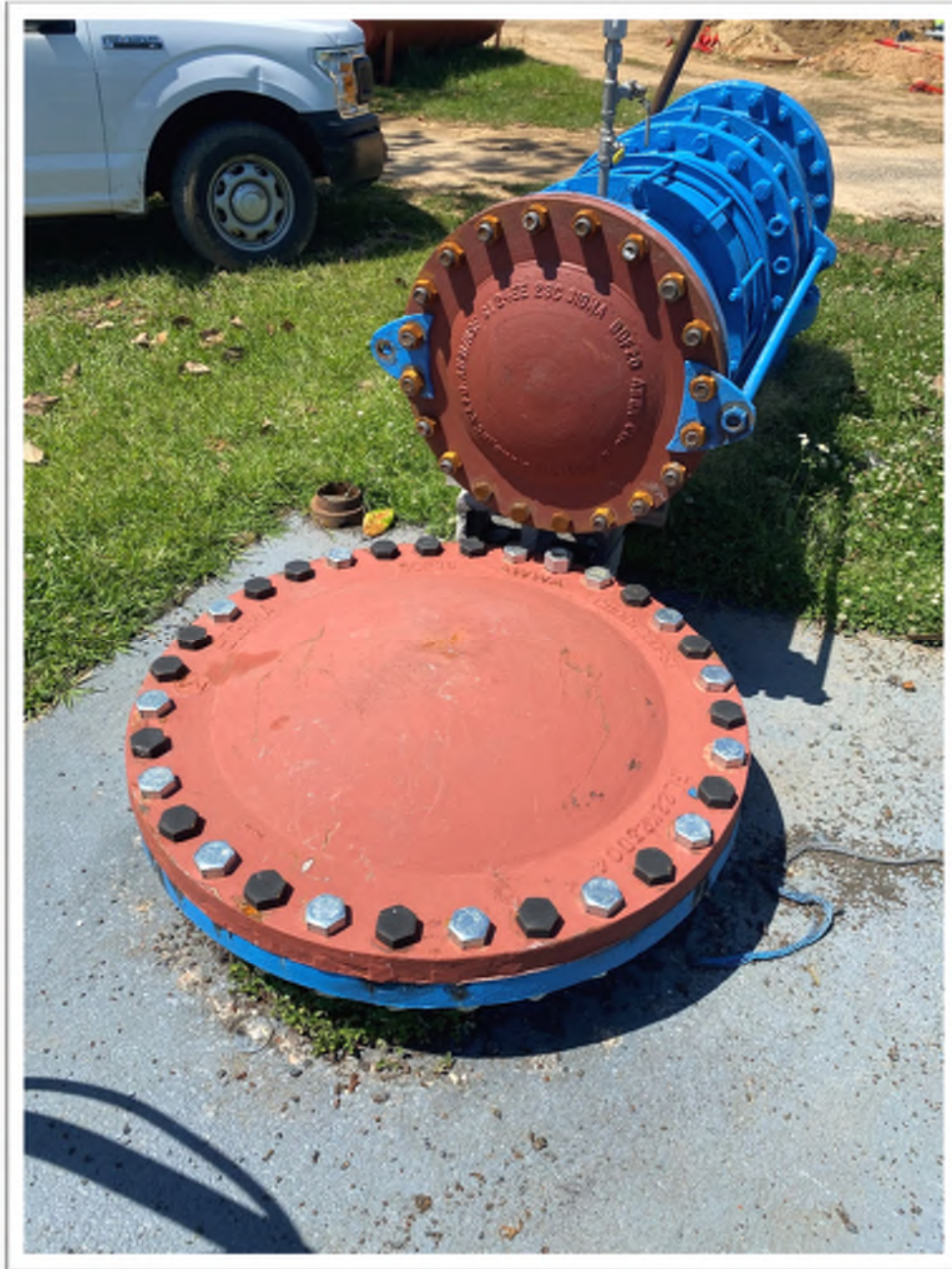
PHOTOGRAPH 1: VERTICAL TURBINE PUMP AND DISCHARGE HEAD INSTALLATION LOCATION (PUMP REMOVED)
