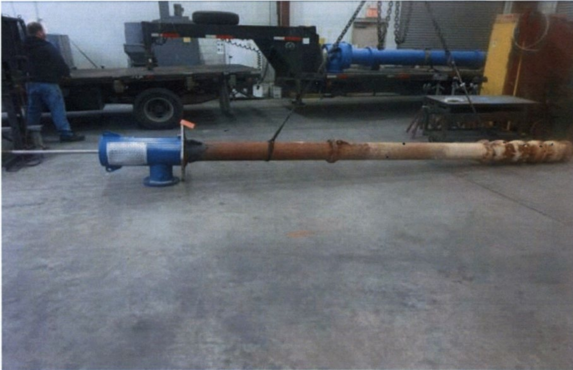
PHOTOGRAPH 2: VERTICAL TURBINE PUMP AND DISCHARGE HEAD (PUMP REMOVED)
