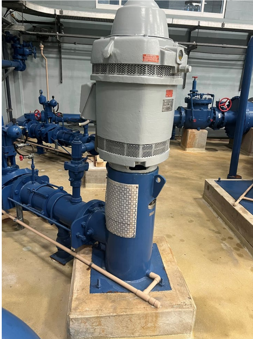
PHOTOGRAPH 1: EXISTING VERTICAL TURBINE PUMP AND DISCHARGE HEAD INSTALLATION
