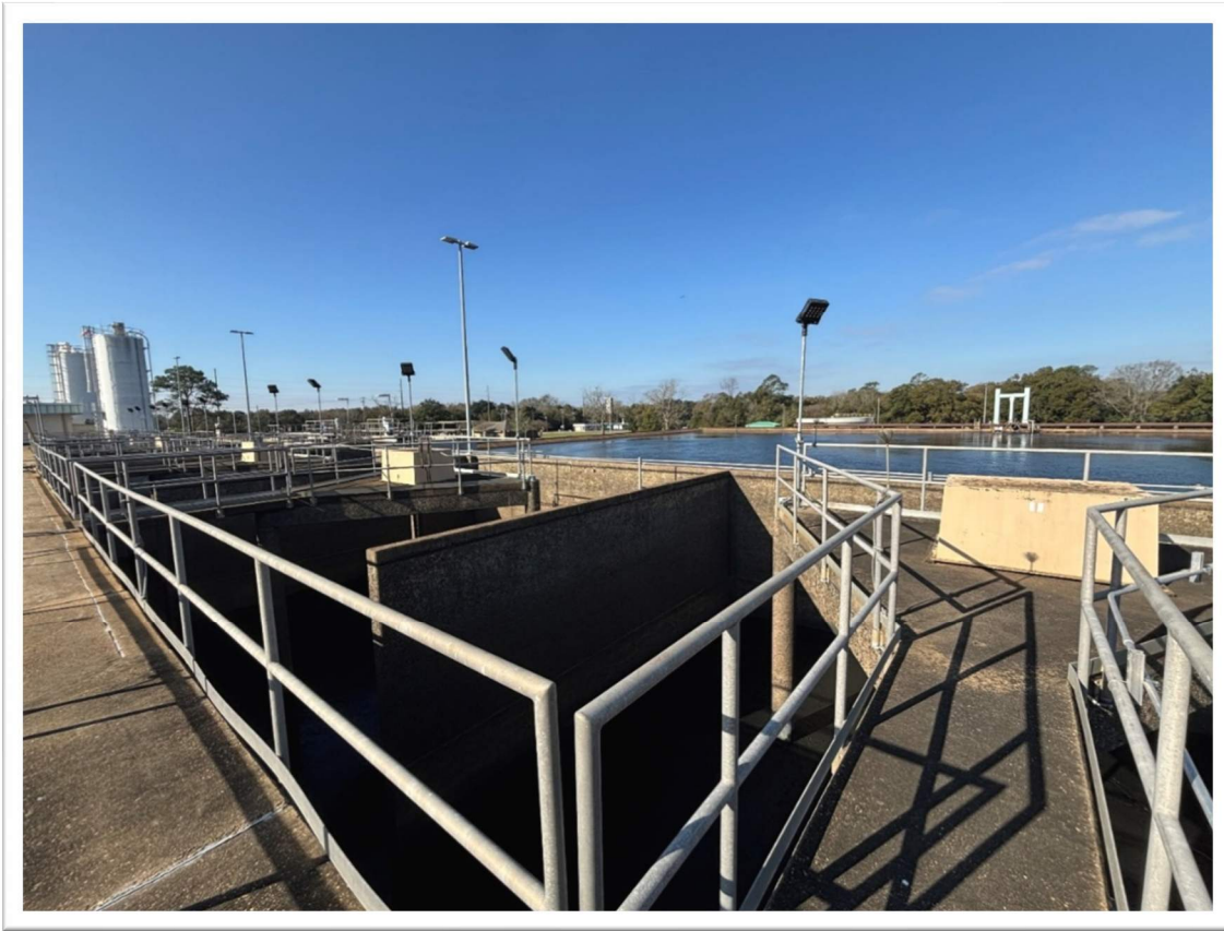
PHOTOGRAPH 1: STICKNEY WTP – FLOCCULATOR BASINS 3 & 4
