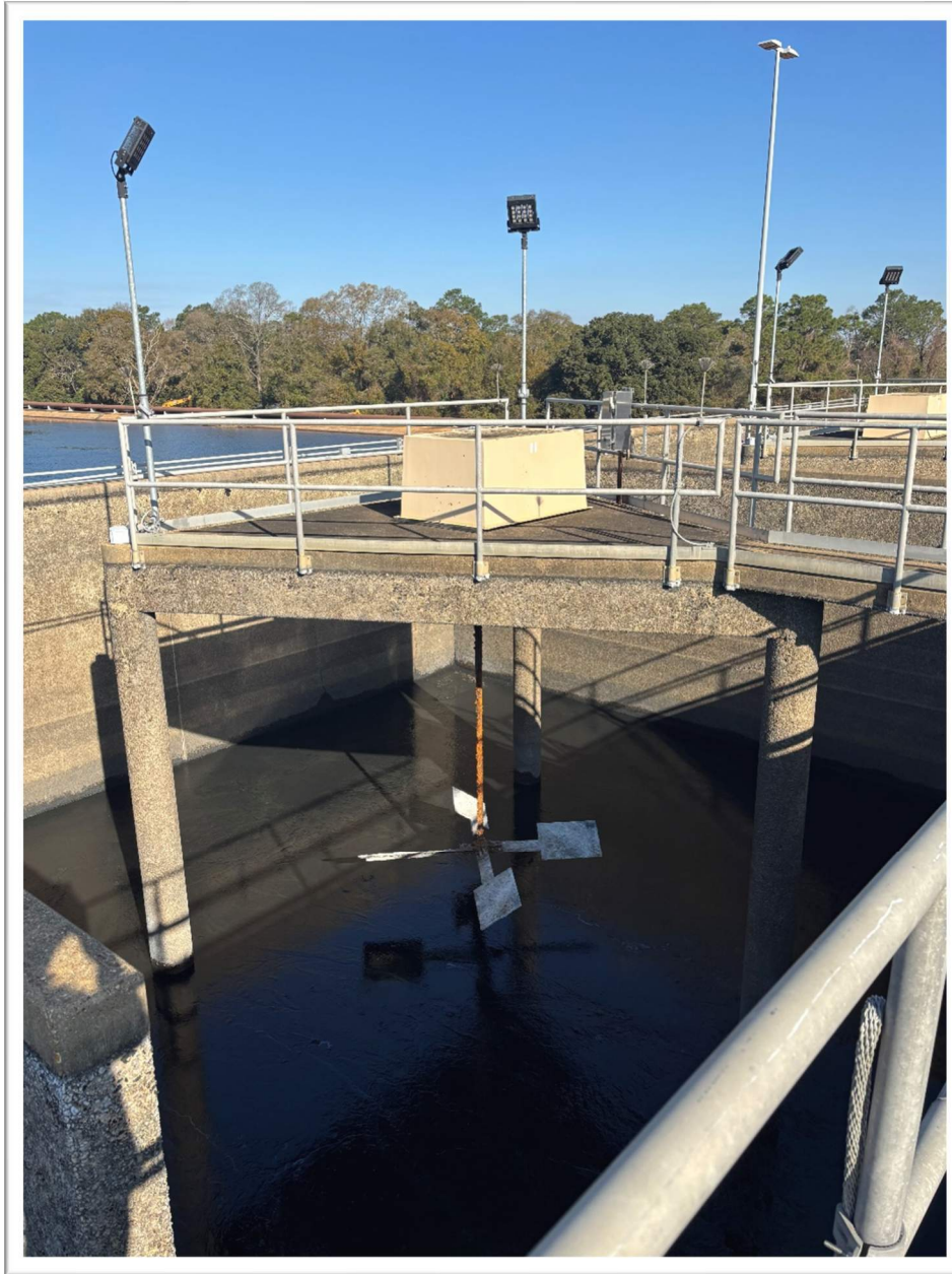
PHOTOGRAPH 2: EXISTING FLOCCULATOR TYPICAL INSTALLATION
