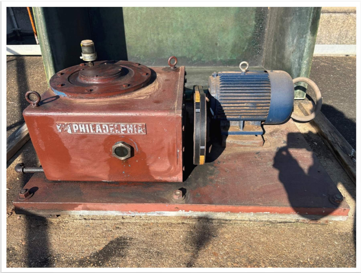
PHOTOGRAPH 3: EXISTING FLOCCULATOR MOTOR AND GEAR REDUCER
