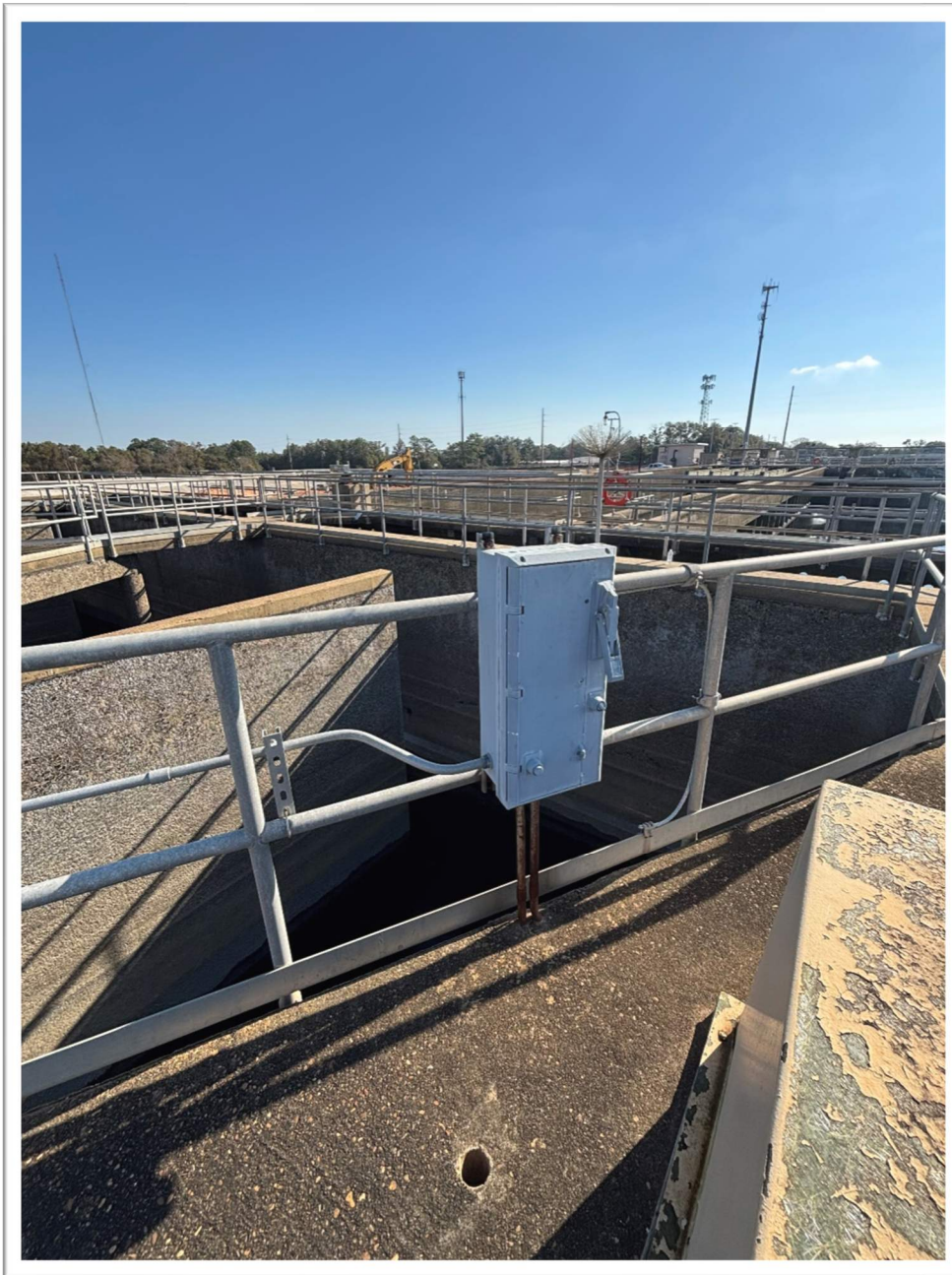
PHOTOGRAPH 4: EXISTING FLOCCULATOR TYPICAL CONTROL PANEL
